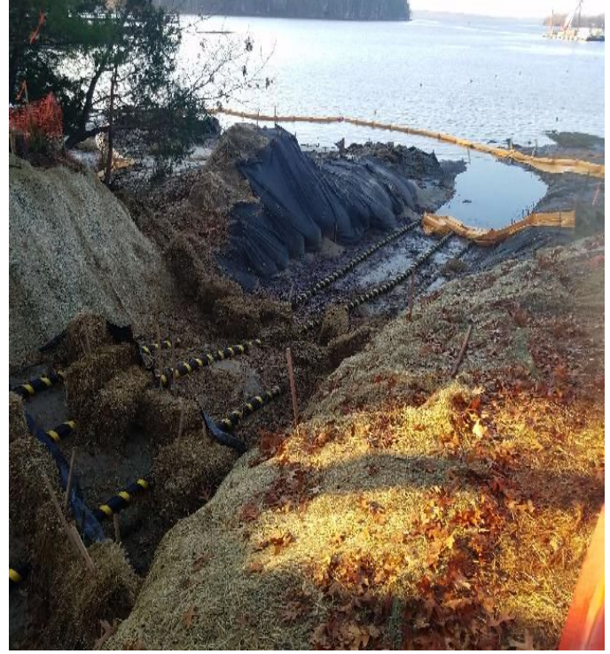
Fig 14: Tide shifted straw bales installed in trench at Gundalow landing /east side of the Bay. (Corrected each day.) Viewing west. (11-25-19).
