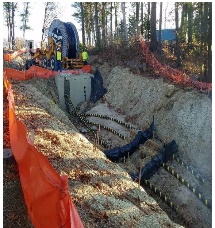
Fig 12: New River Electric Co. positioning cable reel into place at Gundalow landing/east side of the Bay. Viewing west. (11-23-19).
