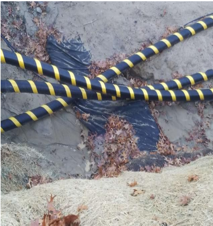
Fig 15: Sediment build up behind sediment controls in trench at Gundalow landing/ east side of the Bay. Viewing south. (11-25-19).
