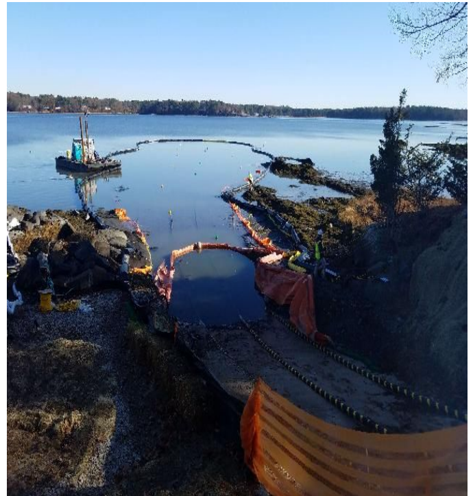
Fig 2: Hand jetting for cable burial at Getchell property/west side of the Bay. Viewing east. (11-21-19).
