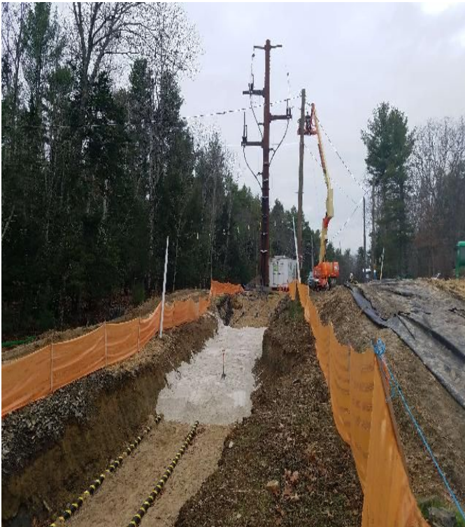
Fig 7: Crew began backfilling thermal sand over cables in trench at Getchell property/west side of the bay. Viewing west. (11-22-19).
