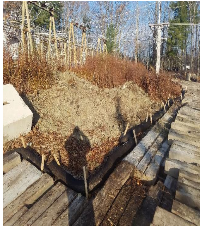
Fig 22: Soil spoils from drilling Str. 1 in uplands with filter sock installed around perimeter. Viewing north. (11-26-19).
