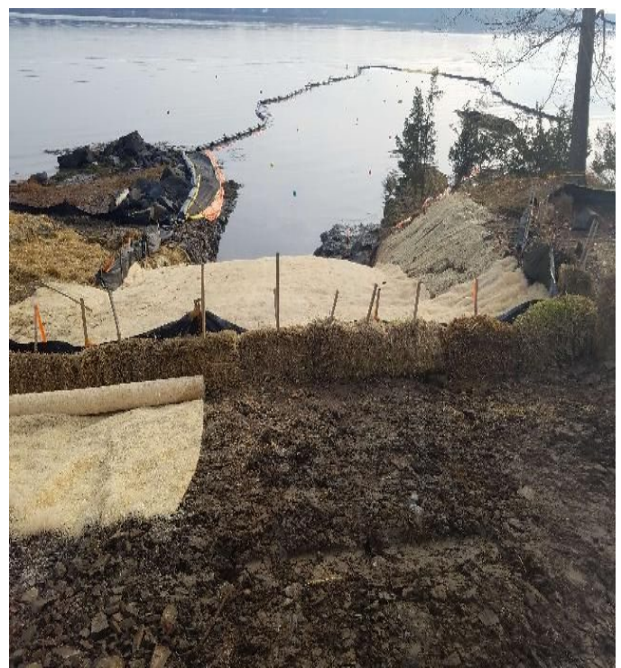
Fig 28: Trench at Getchell property/west side of the Bay backfilled with Temporary erosion blankets installed. Viewing east. (11-27-19).
