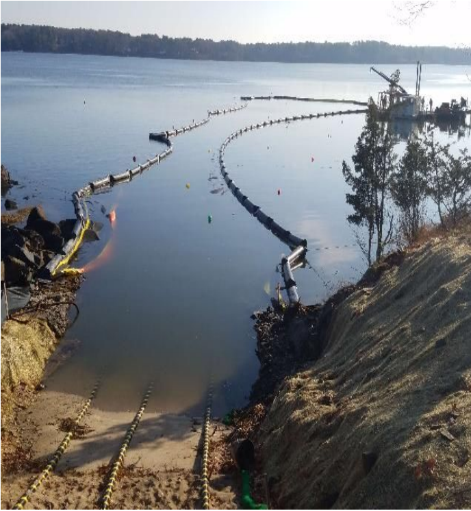
Fig 17: Turbidity curtain shifted at Getchell property/west side of the Bay. Viewing east. (11-25-19).
