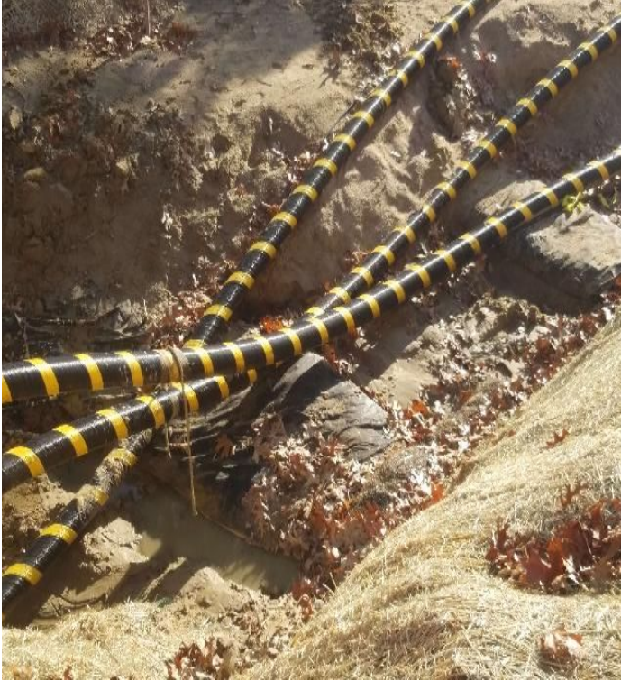
Fig 25: Sediment build up removed from BMPs in trench at Gundalow landing/east side of the Bay. Viewing west. (11-26-19).
