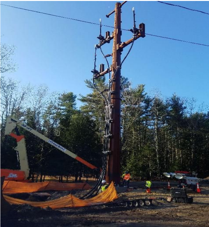
Fig 1: Attaching cable to Str. 99 at Getchell property/west side of the Bay. Viewing west. (11-21-19).
